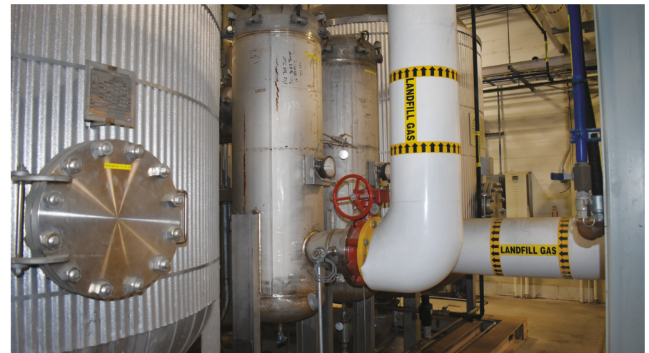
METHANE GAS TO ENERGY FACILITY
